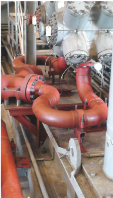
Figure 12: View of longer than optimal PAN pipes before Y-branch.
